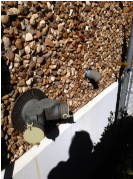
Figure 1.1 FDC (Fire department connection)
